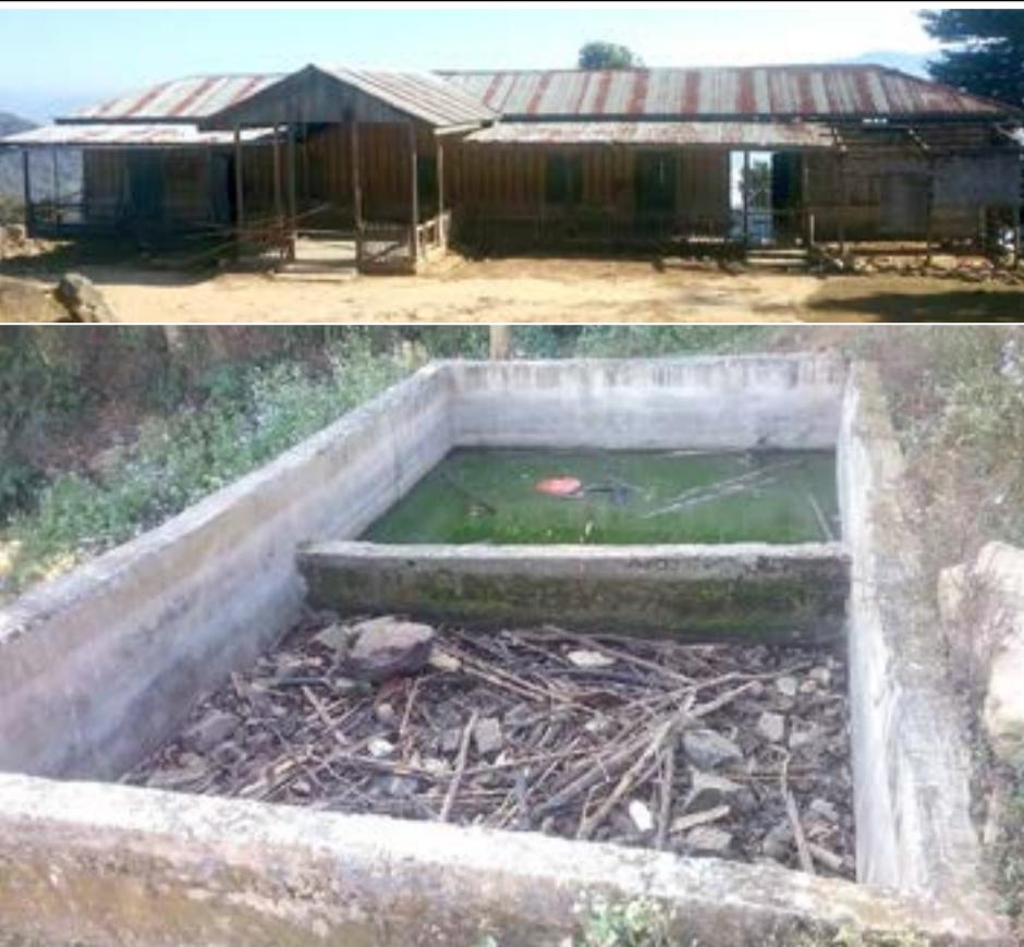
Manipur sawrkarin District thar 7 a puong laia Pherzawl district sunga school building le a bul ela um Septic tank ding ni awm taka siem hman lo le tawp takin a um. Htiengang failed infrastructure hi tam tak hmu ding niin a hmuna zu fe han an hril.
